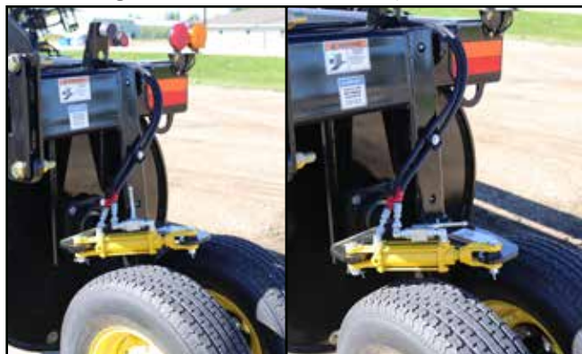
Fig. 46 Steering Circuit Hydraulic Ball Valves: Closed/Open
