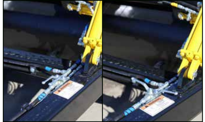
Fig. 64 Hitch Circuit Hydraulic Ball Valves: Open/Closed
